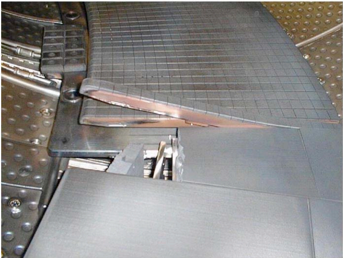
Laplace forces have twisted this element of the Tore-Supra limiter and torn off its carbon covering
