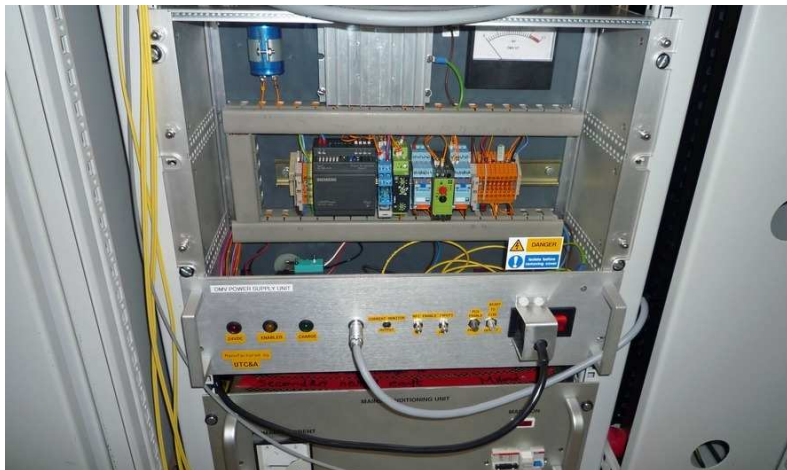
Figure 5.11: DMV power supply located in 19 inch cubicle. The front panel shows various status indications and interlock connections. The red, green and yellow lights (lower left corner of image) indicate the presence of mains power, the presence of the control system enable and the start of charging respectively.
